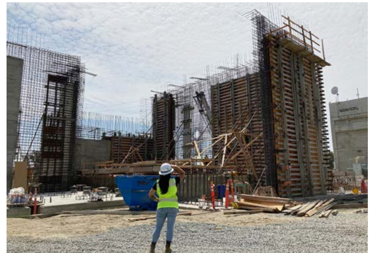
Construction of low flow pump station at Plant No. 2 in Huntington Beach.
